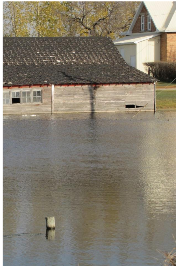
Fig. 13 —High water tables that are further exacerbated by heavy spring run-off can present significant challenges (M. G. Miller, 2011)
