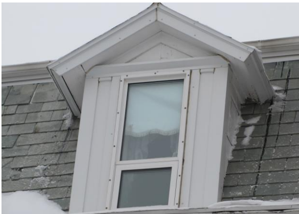
Fig. 5 — The installation of aluminum or PVC windows where wood windows existed historically results in material incompatibility (Photo: M. G. Miller, 2010)
