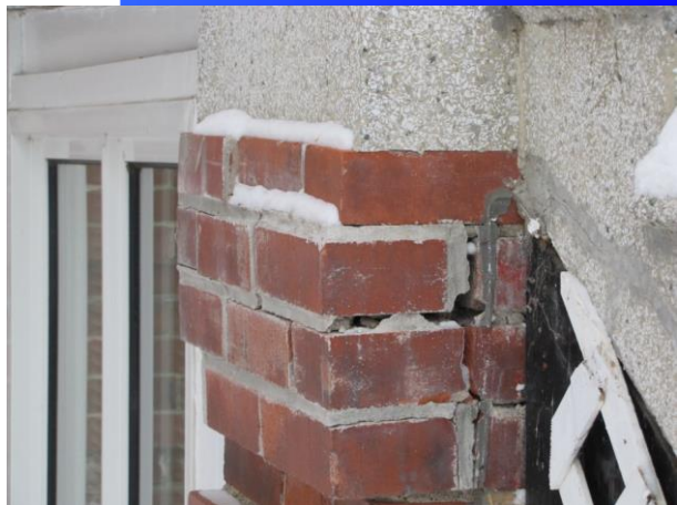
Fig. 3 — Inadequate maintenance in the form of deferred re-pointing or the use of incompatible mortars can accelerate deterioration (Photo: M. G. Miller, 2010)
