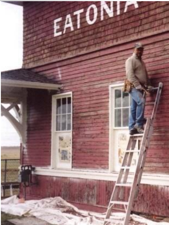
Fig. 15 — Hand-scraping and the selective repair of historic siding is an appropriate conservation approach (M. G. Miller, 2011)
