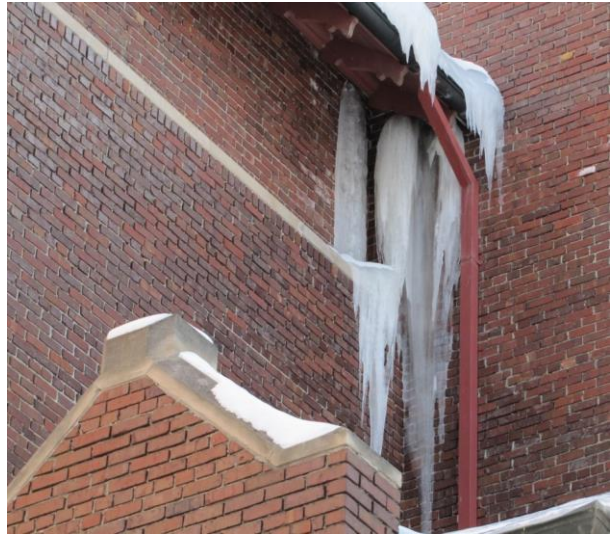
Fig. 12 —Ice-damming in areas that are not easily accessible can present a challenge (M. G. Miller, 2011)
