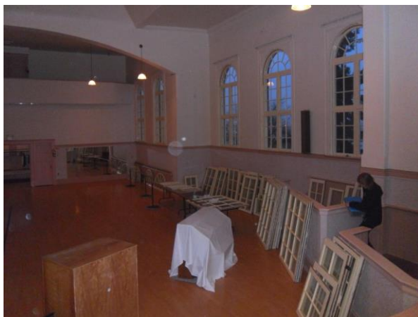
Fig. 6 —Repairing and selectively replacing extensively deteriorated component sash parts represents best conservation practice (Photo: M. G. Miller, 2010)
