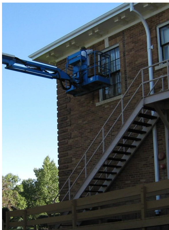
Fig. 2 — Re-pointing historic masonry with compatible mortar is an effective conservation measure (Photo: Town of Shaunavon, 2010)
