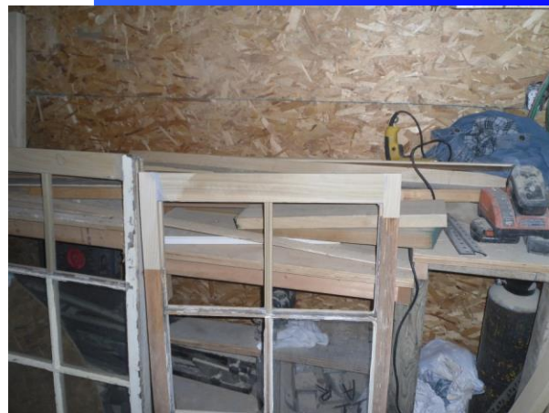
Fig. 7 —In-kind splicing of new wood to match existing represents best conservation practice with regard to extensively deteriorated sash components (Photo: M. G. Miller, 2010)
