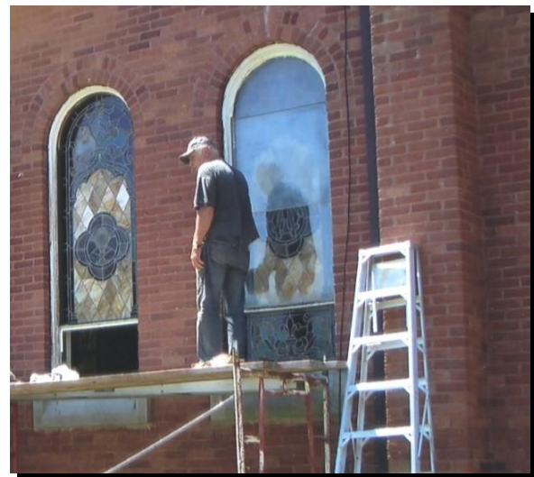
Marysburg RC Church, SK A Lexan storm window will protect the stained glass from breakage caused by rocks, hail, and birds, but has a major visual impact on the building. Although Lexan is clear and very reflective when first installed, it will pit and become almost opaque within a decade.
