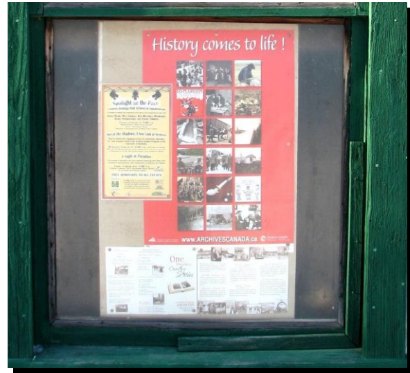
Former Dollar Land Co. Office , Truax SK The Lexan in this window is so pitted and yellowed that it is difficult to read the display.
