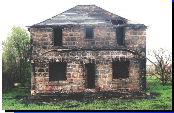
Kerrobert Area Residence Damaged by Fire RM of Mariposa, SK
