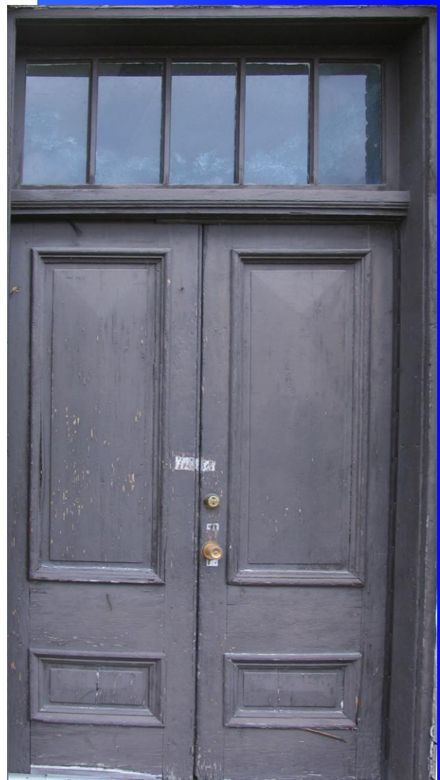
Fig. 14 — Raised-panel timber-frame doors with multi-light transom, McNaughton Stores building (1890) (Photo: M. G. Miller, 2011)
