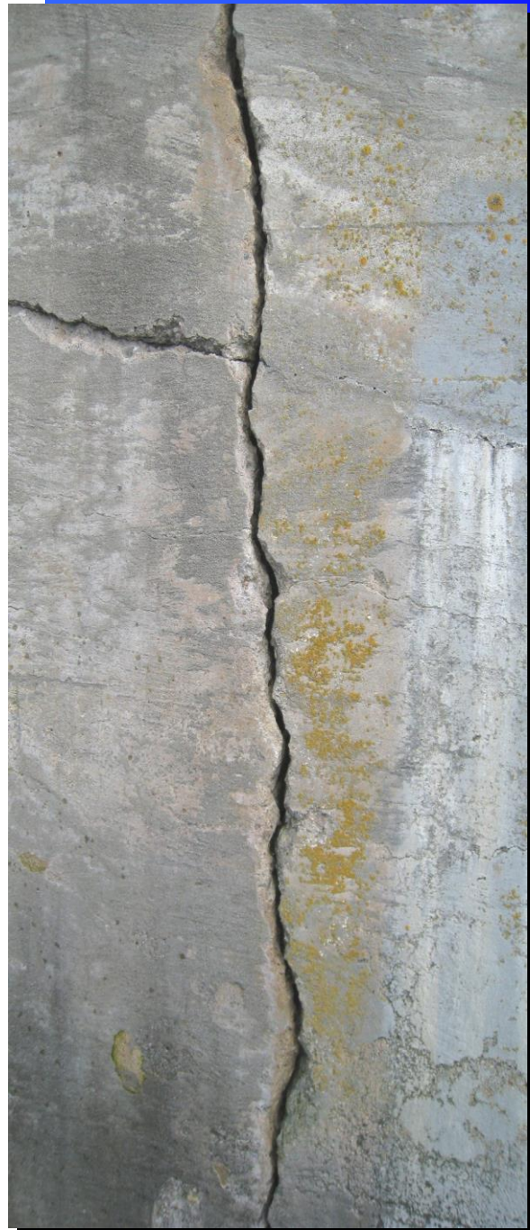
Typical Vertical Foundation Cracking / Zelmer
