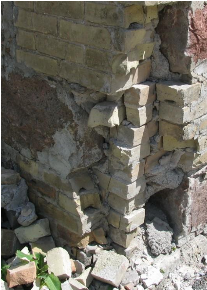
Fig. 29— Dislodged masonry at the 1886 McNaughton Stores in Moosomin.
