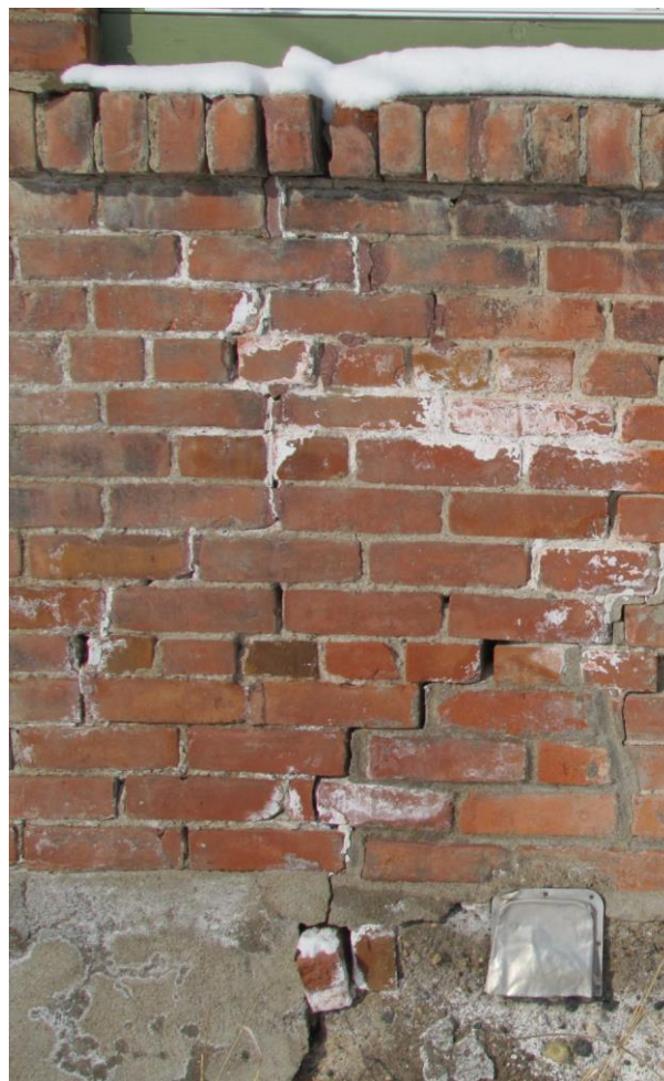
Fig. 15— Soiling and efflorescence at The Stoop, Rouleau
