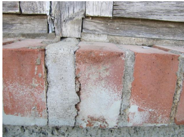
Fig. 19—Mortar joints at the Veteran's Memorial Hall in Earl Grey.
