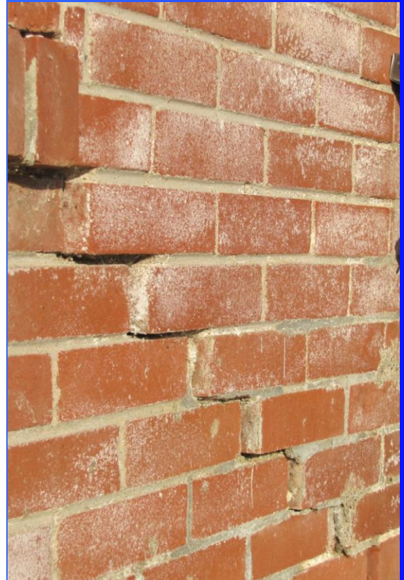
Fig. 13—A masonry wall shifts out of plane at the Veteran’s Memorial Hall in Earl Grey.
