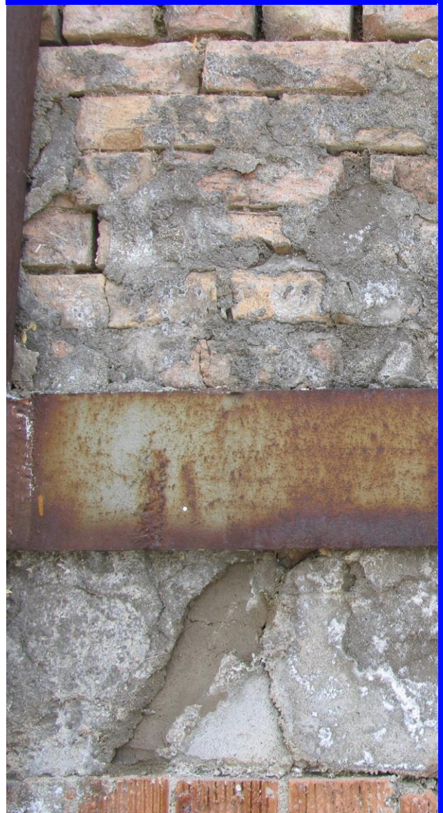
Fig. 18—Previous masonry repairs at a kiln at the Claybank Brickplant, National Historic Site.
