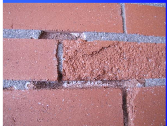
Fig. 14—Spalled masonry unit at Khedive Recreation Centre, Khedive.
