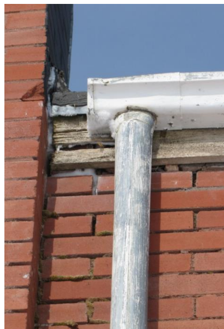
Fig. 6—Masonry damage at a common point of failure at the Khedive Recreation Centre, Khedive.
