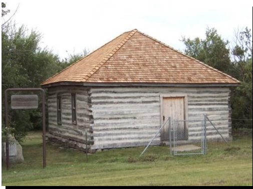
Shiloh Baptist Church, erected NE of Maidstone in 1912, was restored in part from assistance provided by the J.M. Kaplan Fund, which focused its funding primarily on rural churches.
