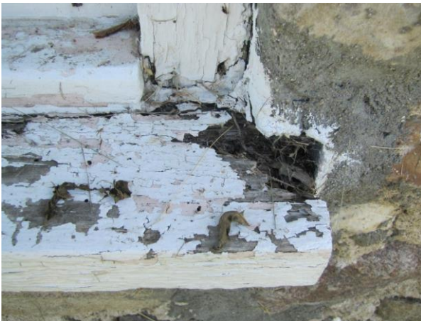
Fig. 4 — Timber sill showing effects of moisture entrapment, Stone Church, Wishart (M. G. Miller, 2011)
